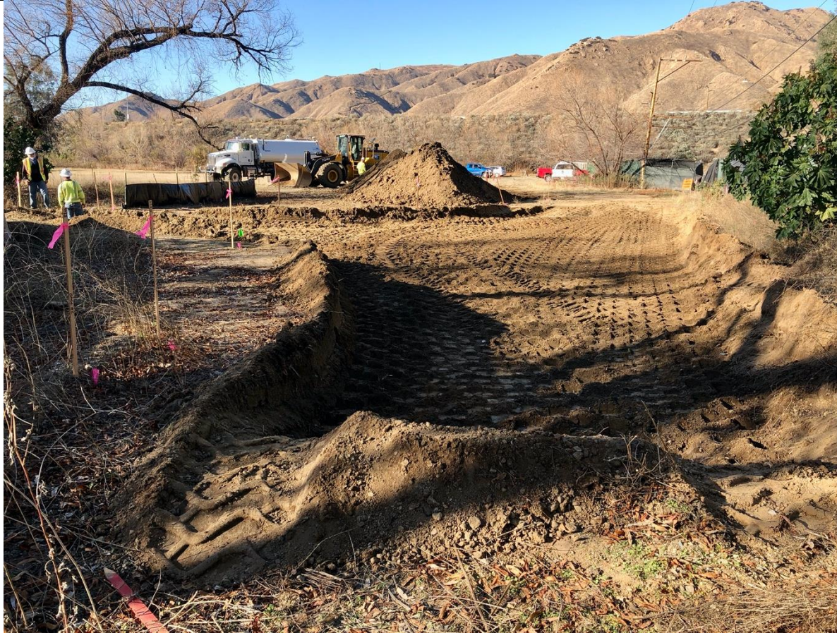
Photo 4 – Access road enhancement at TSP site 522. BMPs are in place. Photo facing northeast
